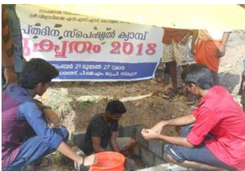
Compost pit side wall work by NSS Volunteers at PJM UP School
